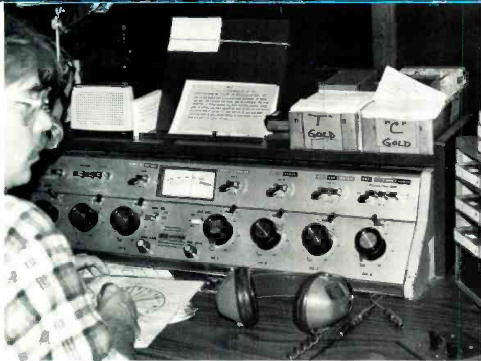
WKOP's control room has a Gatesway 80 board and an ITC 3D cart machine. One of the challenges of moving into the new facility was that no new equipment was purchased.
