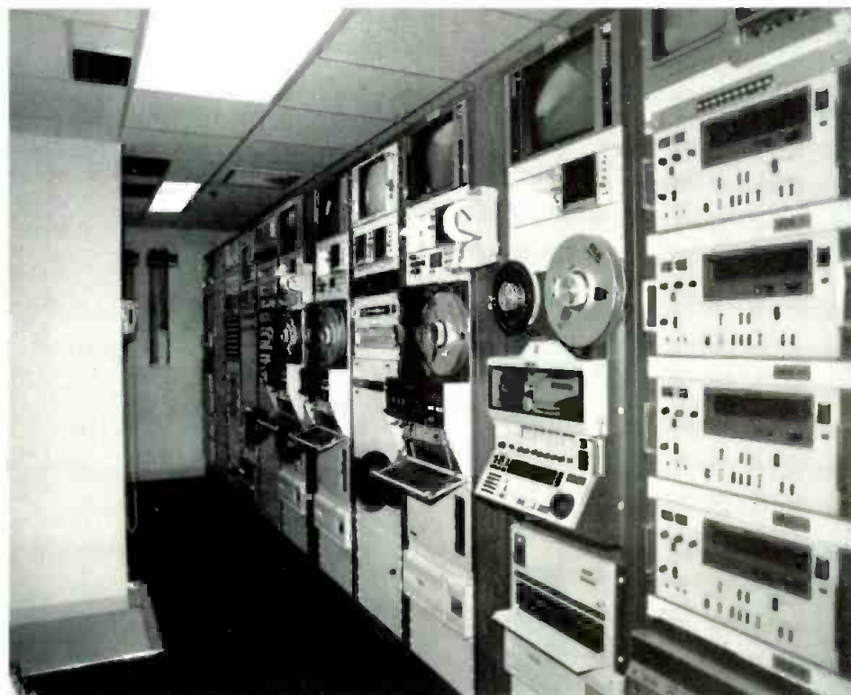
The equipment room, with one row of 11 racks, offers monitoring, taping, patching, and time base correction. The tape machines shown here are a Sony BVH 2000, and three Ampex VPR 2Bs.
